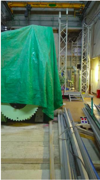
15.5.2018 Emergency Diesel Generator cover wet
