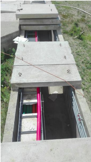
15.6.2017 outside cable canal, open for month, dirt entering
