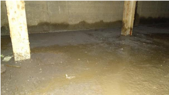
12.1.2018 Room 568 / 1-02, water in basement of canal
