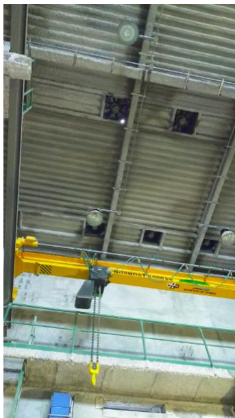
15.5.2018 DG building, hole in roof
