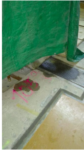
15.5.2018 Emergency Diesel Generator wet patch
