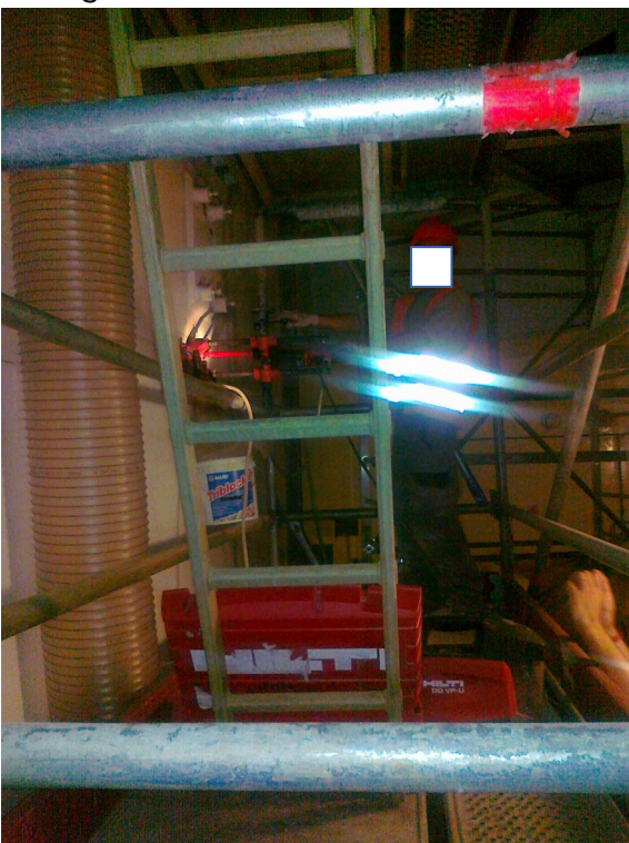
Diamond core drilling (for Hilti mechanical anchor, drilling of much bigger diameter without test drilling was also common according to the witness) (2011)
