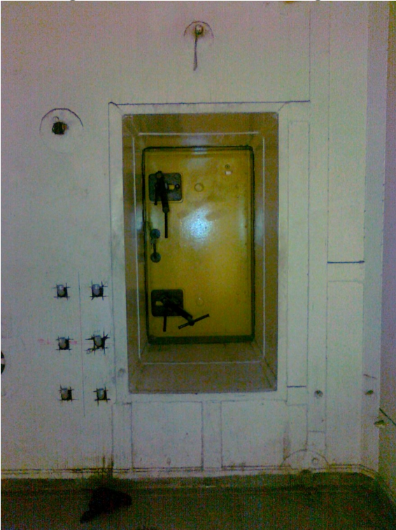
Additional anchors set through steel lining before installing an anchoring plate, without test drilling
